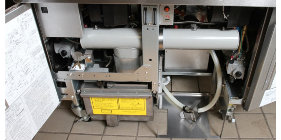
Figure 1: The fryer prior to the install is show above. The sensor mounts on the channel behind the center upright. The pre-filter mounts above the filter pan pickup .
